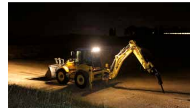
Excellent lighting for night working
