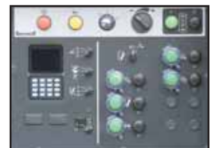
Main control panel
